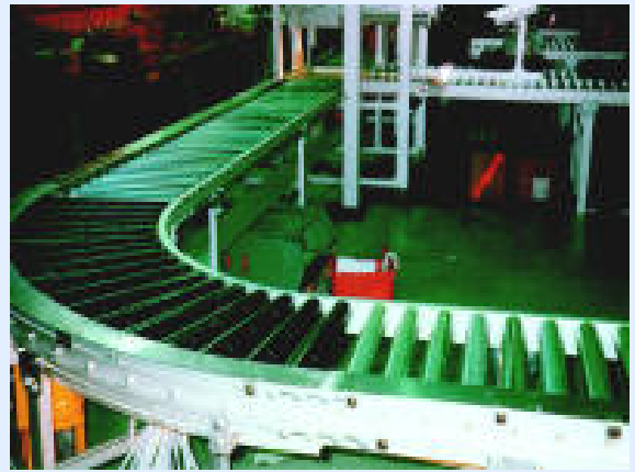
Roller conveyors combined with belt conveyors, stops and pusher stations.
