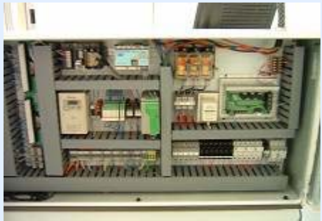
Electrical Enclosure for Automation Process
